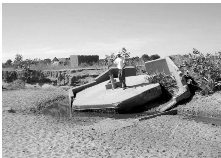
Figure 5: Total collapse of well infrastructure due to seasonal flood erosion, near the village of Abdi in eastern Chad. This can be prevented by locating production wells outside of a wadi, along fractures fed by the wadi's deep reservoir.
